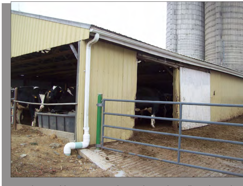
A roof gutter and downspout connected to an underground pipe collect and carry clean water away from this animal concentration area.
